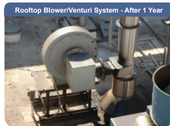
The venturi systems with blowers mounted out of the process stream are mounted on the roof. After 1 year installation there is still minimal oil carryover.
