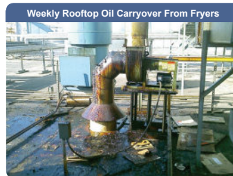
The fryers were vented straight to the roof, and enough oil collected on the roof to require weekly cleaning, and cause environmental concerns.
